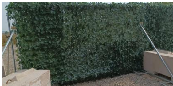
Plate 3.5 Heras fencing with attached textured plastic hedgerow
